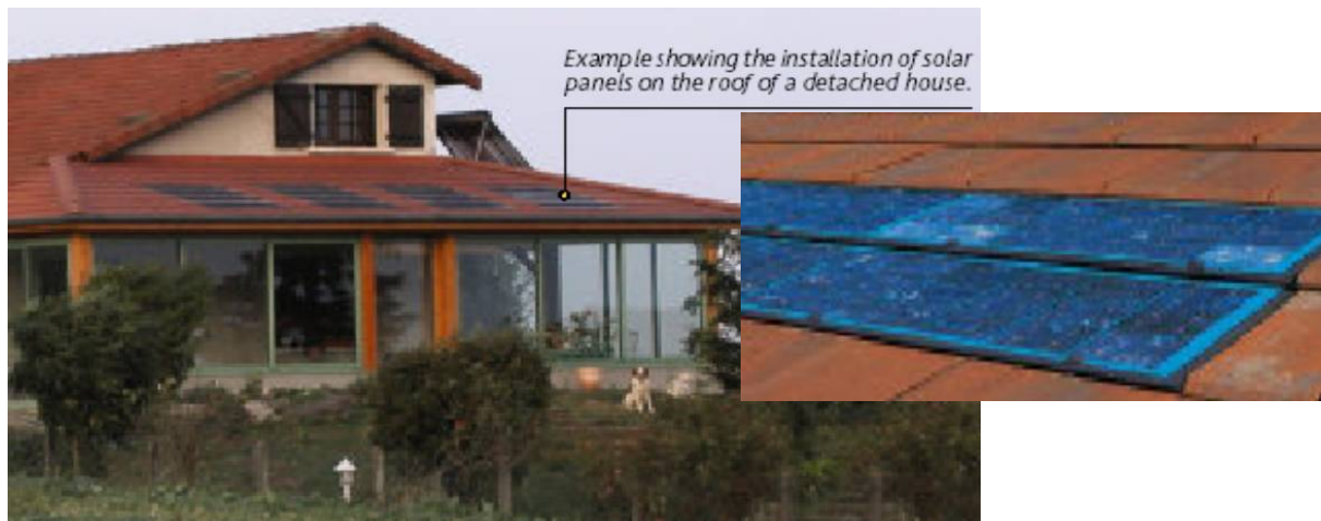
Fig. 2.4: Picture of the F1 PV system near Lyon and its PV roofing tiles.
